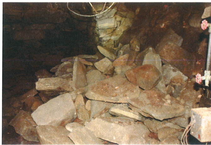
PHOTO #2 - Fallen Stone
