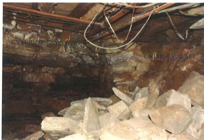
PHOTO #1 - Wall & Fallen Stone
