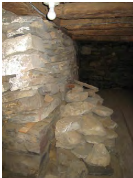
Photo 1 Failing foundation wall, east side of chimney (Facing north, toward Middle Road)
