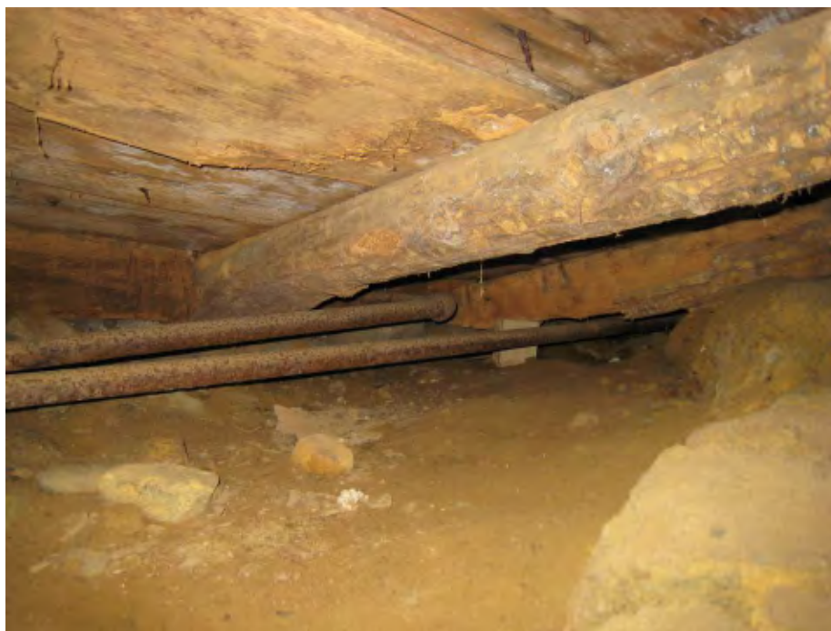
Photo 5 Collapsed first floor framing section (Facing north/Middle Road, center section north of chimney as viewed from crawlspace)
