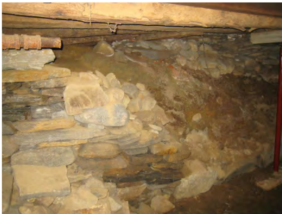
Photo 2 Failing foundation wall, west side of chimney (Facing east, toward driveway/parking area)
