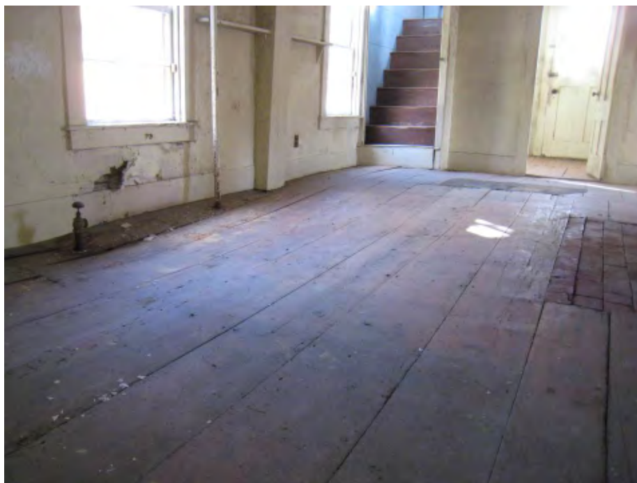
Photo 6 Collapsed first floor framing section (Facing northeast/Middle Road, center section north of chimney as viewed from first floor)
