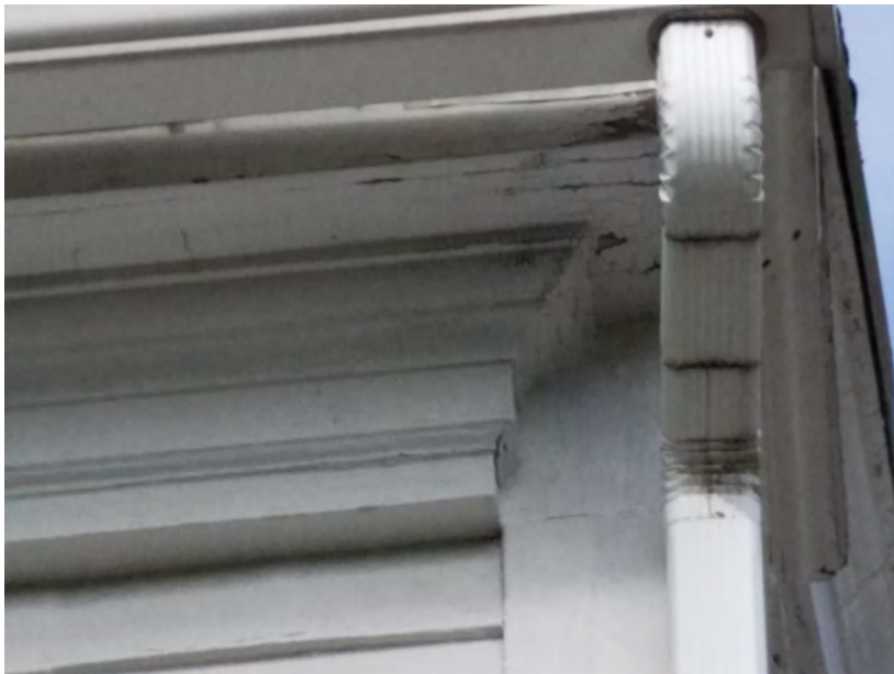
Condition at southeast cornice return. Note cornice below soffit.
