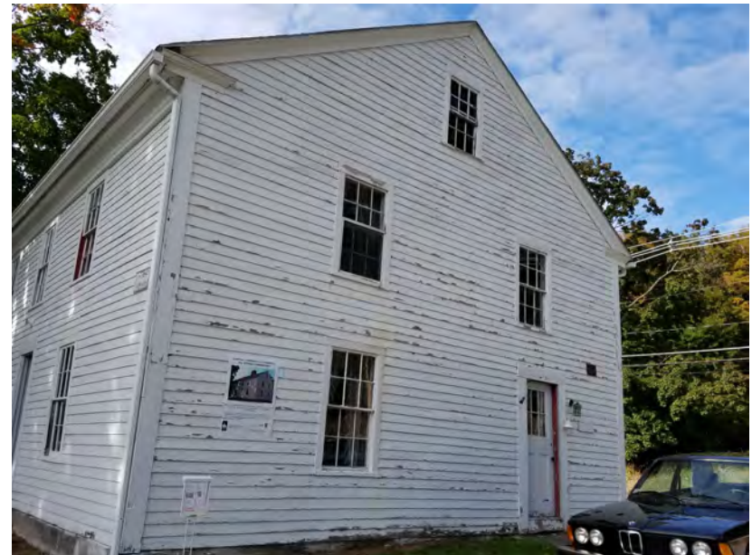
Typical condition of paint. East side shown.
