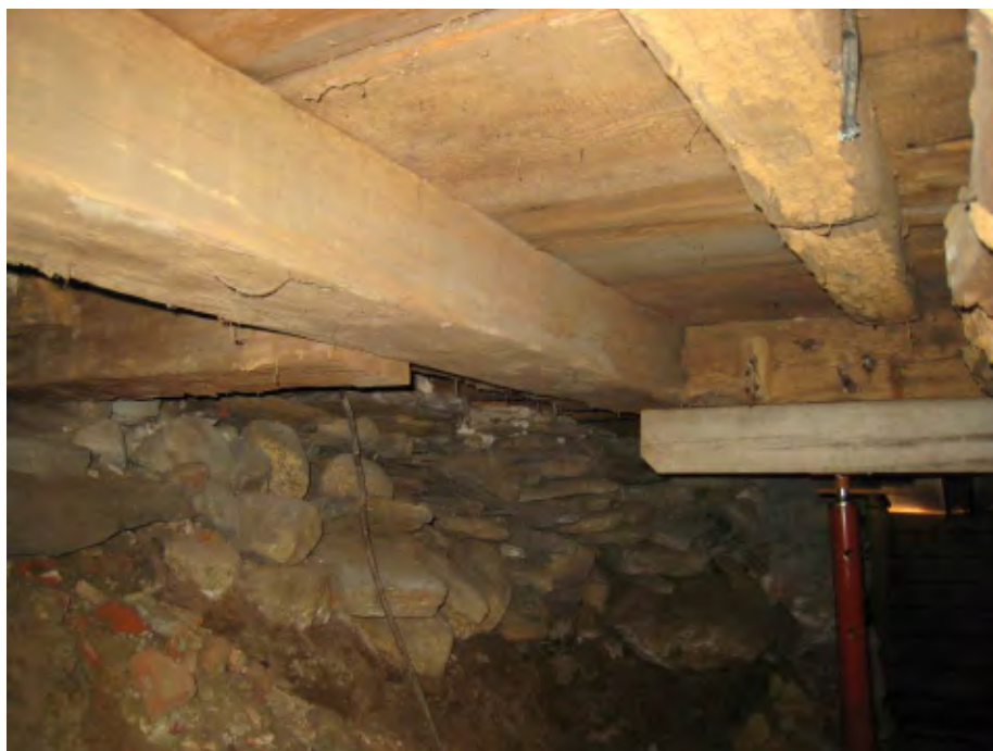
Photo 3 Beam previously supported by now-collapsed chimney wall (Facing south, toward barn)
